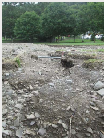
Electric lines in conduit trenched in on Monday of last week and exposed on Monday of this week.
